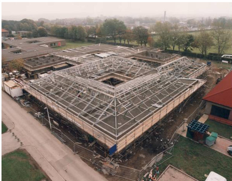
Figure 1 Over-roofing of hospital building using long span Capella roof trusses from Kingspan
